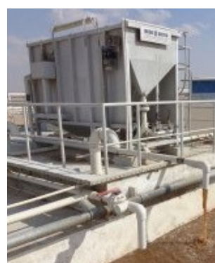
Industrial ETP Plants (Industrial Effluent Treatment Plants)
