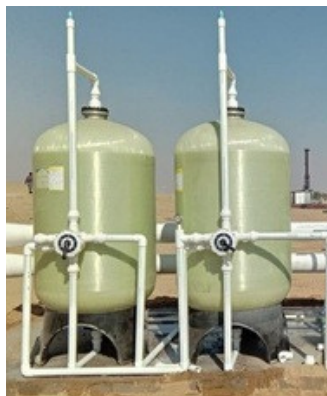
WTP PLANTS (Water Treatment Plants)
