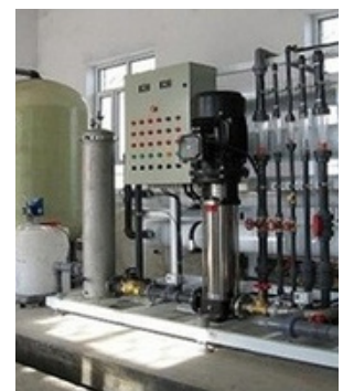
INSTITUTIONAL RO PLANT
