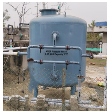
WTP PLANTS (Water Treatment Plants)
