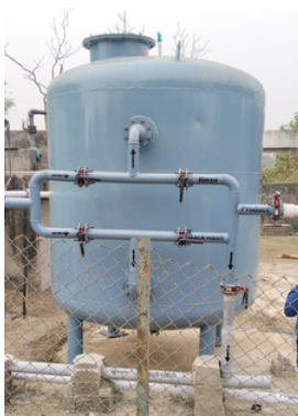
WTP PLANTS (Water Treatment Plants)
